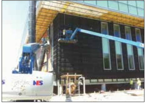
Vertical rails are attached to clips welded to the building's steel girders.
